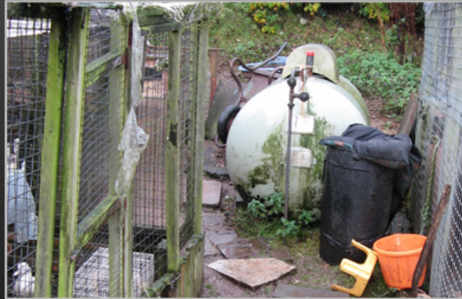
Poorly-sited tank with clutter around it
