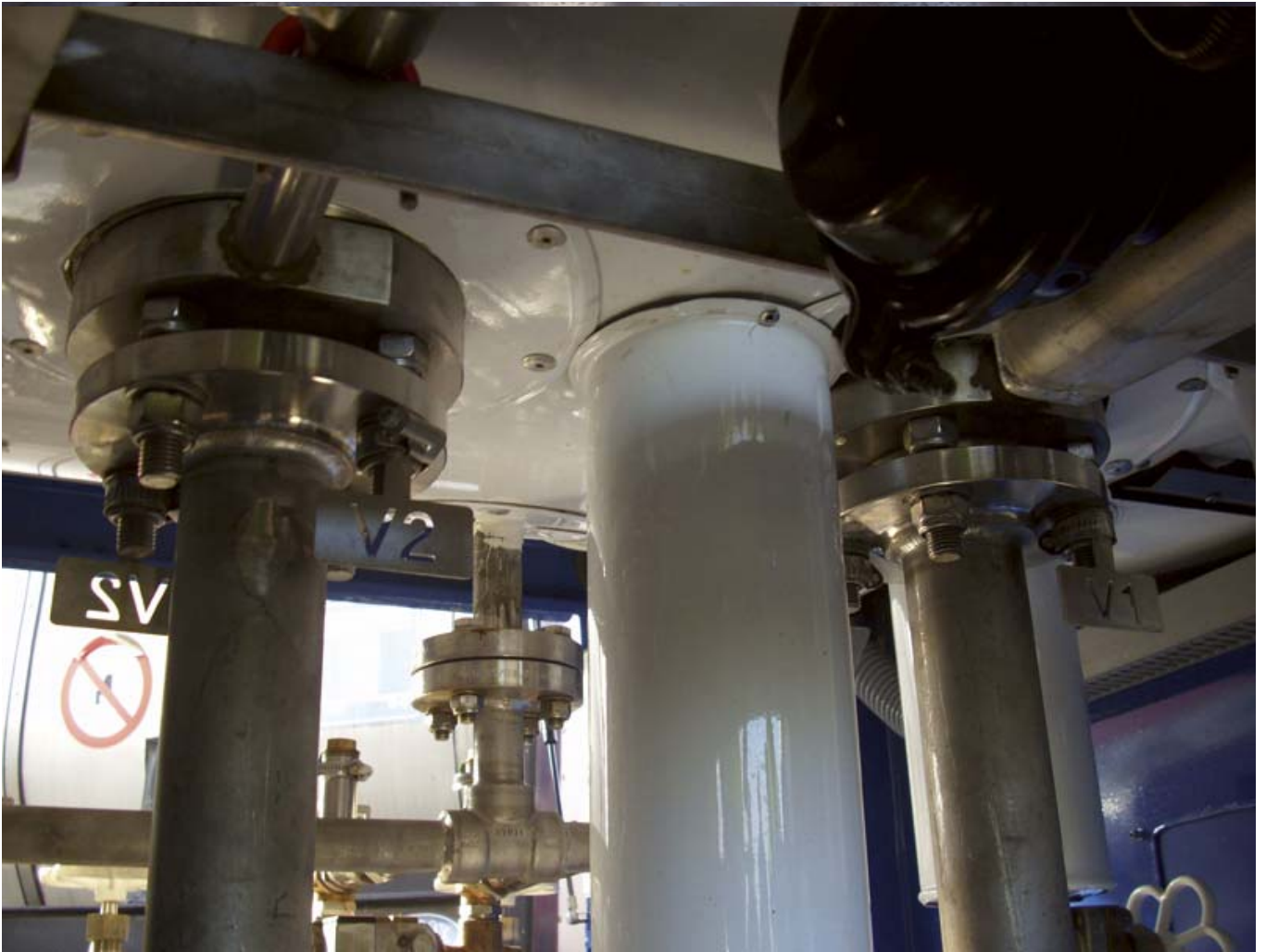
Figure 7. General view of the set of valves and pipelines. In the foreground, the loading and unloading connections. The right-hand photo shows a detail of the inner plug valves. Source (4) : Authors.
