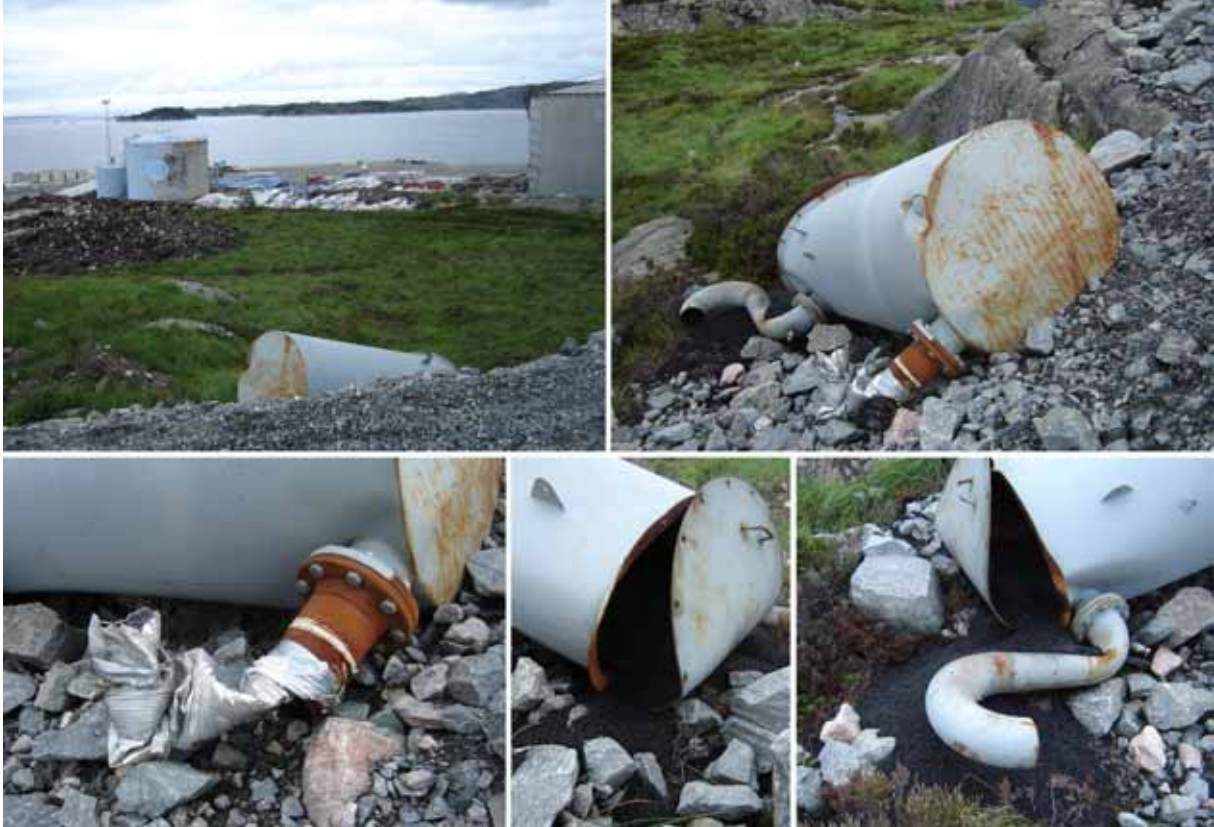
Figure 6-3 The air filter from tank T3: position in the terrain (above), inlet with the remains of the flexible pipe (lower left), the lid on top of the filter (lower centre), and the outlet from the filter (lower right).
