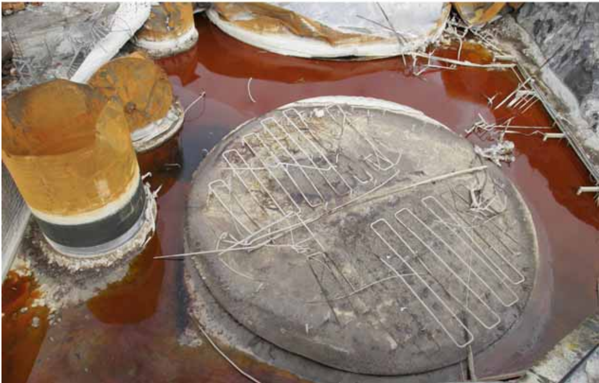
Figure 3-2 Tank farm II viewed from the south (pictures taken from the roof of tank T2, see Figure 1-2). The upper picture shows the three smaller tanks C1-C3 along the bund, the upper part of T3 thrown partly out of the tank farm, and T4 collapsed; the base of T3 is below the water (The Norwegian Police, 25 th May 2007). The lower picture shows the base of tank T3 with the heating system (The Norwegian Police, 31 st May 2007).
